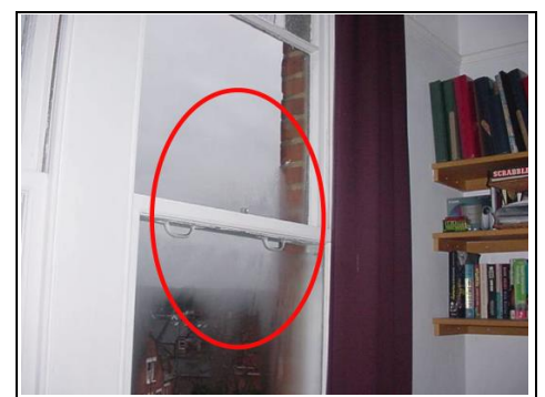
Window with condensation
