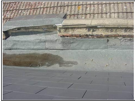
Lack of any decent flashing at all to the middle and front of the right hand valley gutter
