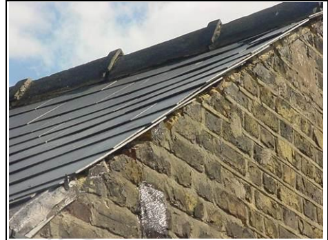
Close up of flashing put on incorrectly
