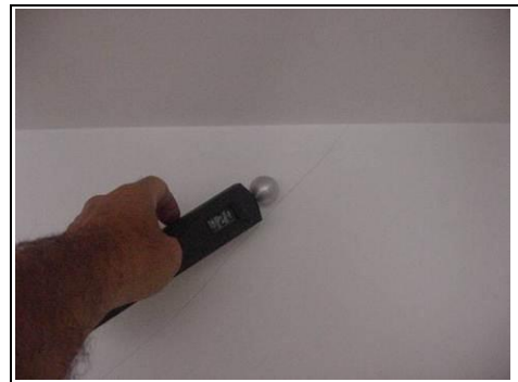
Hairline crack with reading of 28
