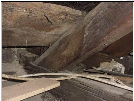
Staining on the timber that is typical from what you see from a leaking valley gutter
