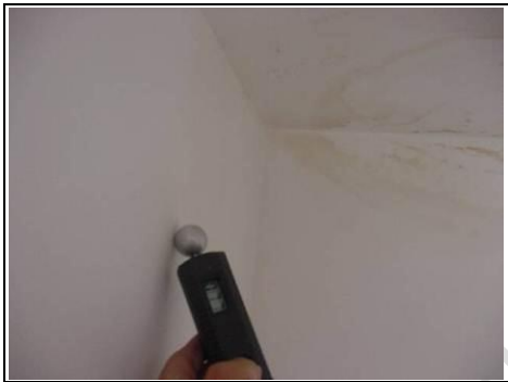
Damp meter reading of 77
