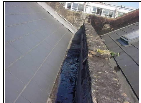
The parapet wall that is allowing water in. This explains the plant growing out of it. This needs to be made watertight
