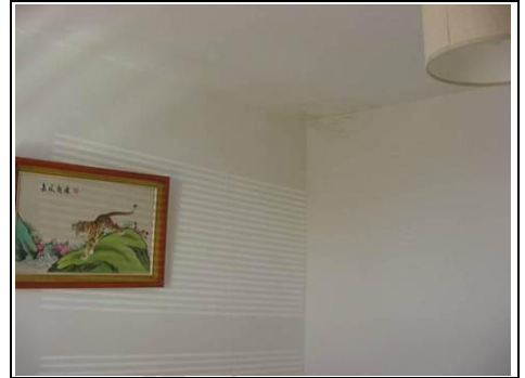
Dampness in the corner of the rear bedroom
