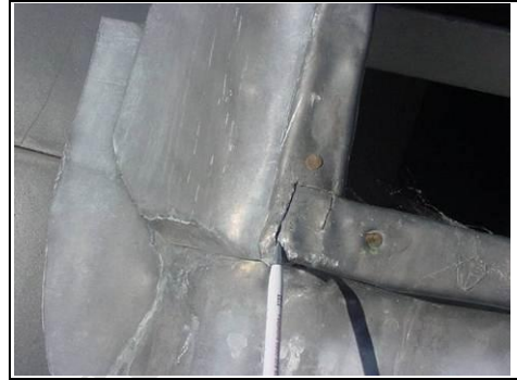
Damage to the lead
