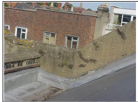
Flashing not fitted correctly to the front right hand side
