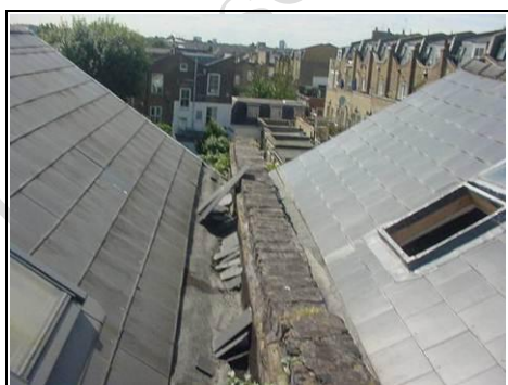
Many slates have been damaged
