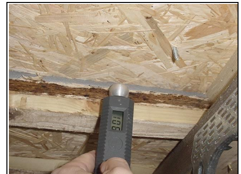
Damp meter readings underside of the gully
