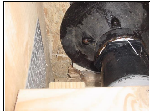
Rusting to bottom and screws
