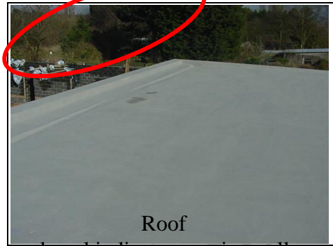
Roof red oval indicates running gulley
