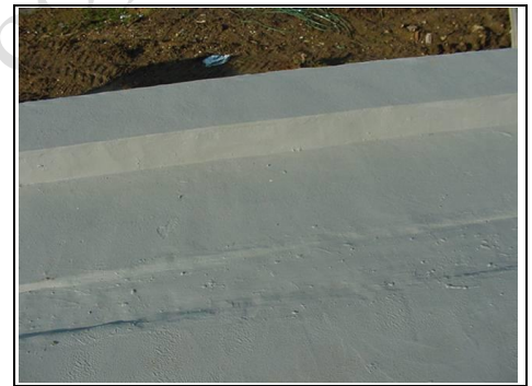
Stippling/puckering to roof surface
