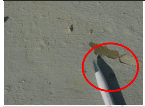
Close up of area of surface coming away
