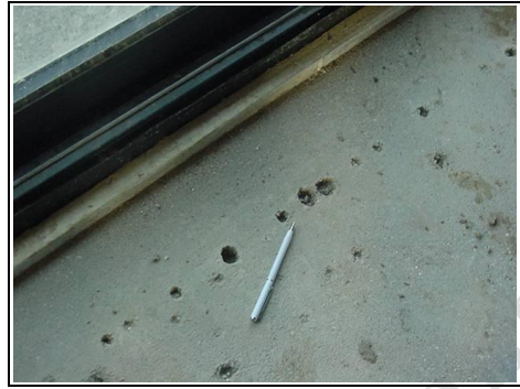
Pattern staining Rear right
